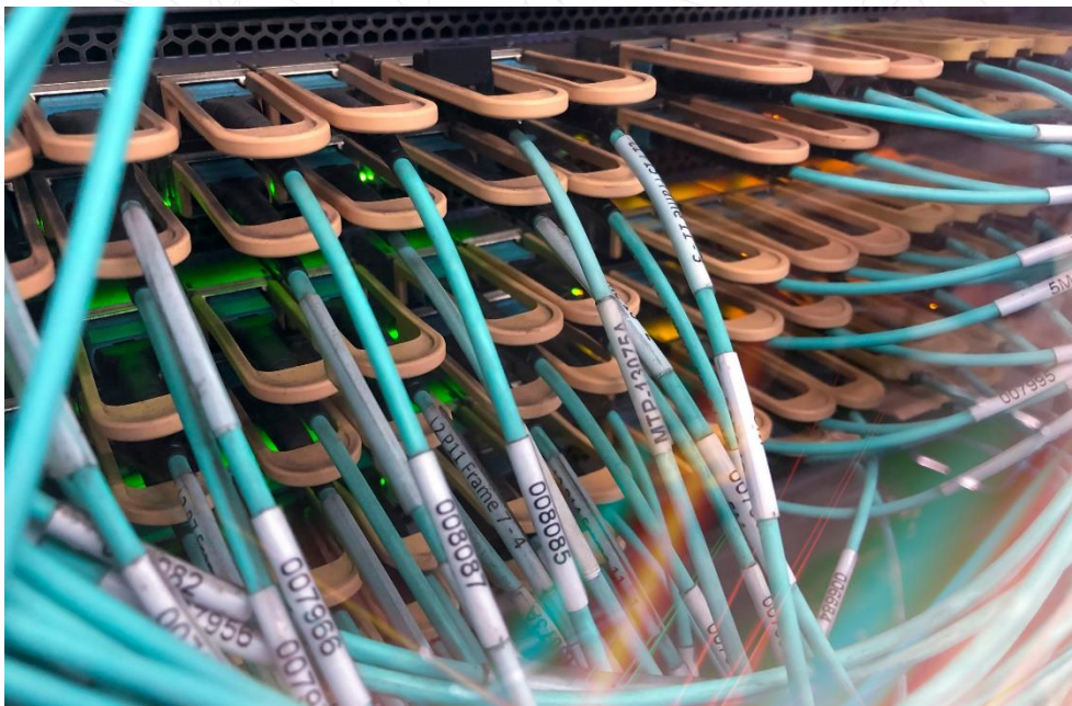
Figure 1: QSFP transceivers plugged at high density into several optical switches on racks.
